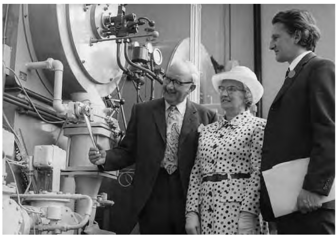
James Cropper with retiring Chief Engineer Jim Hill and Mrs Hill by one of the new gas and oil fired boilers, 1974.
